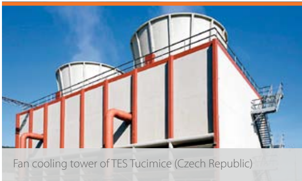
Cooling tower of Pocherady TPP
